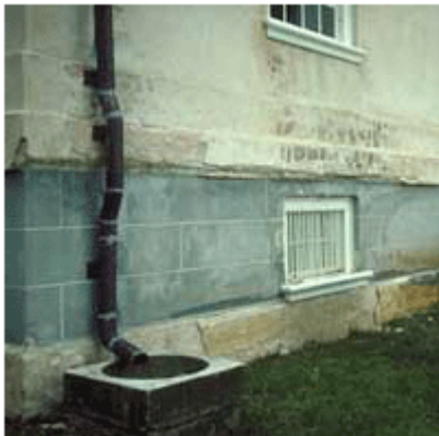
The damage to this stucco appears to be caused by moisture infiltration.
