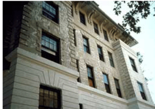
Caulking is not an appropriate method for repairing cracks in historic stucco.
